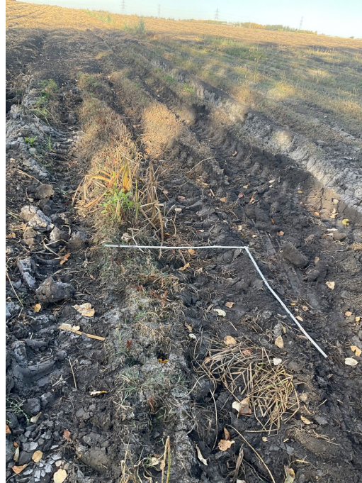
Appendix Photo D-5. View of west showing rutting within the Bypass footprint in a temporary graminoid marsh wetland (WL-28), September 28, 2023.
